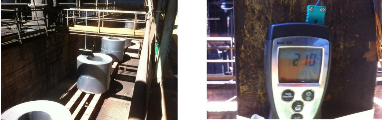
Figure 4: a) Coil in the Conveyor b) Punctual temperature measurement
